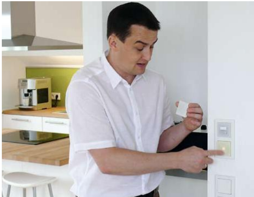
In the Wetzlar Digitalstrom apartment, Lars Wilhelm of aizo presents the various possibilities of the new technology. Photos Richard Staub
